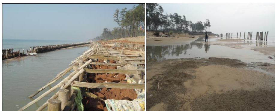
Photo No-1 : Narrowing beach width and exposed mud bottom along the chandpore coast
